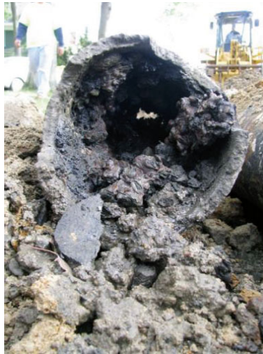
Old Unlined Cast Iron Water Main Pipe
