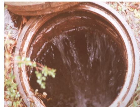
Inflow into a Manhole during Flooding
