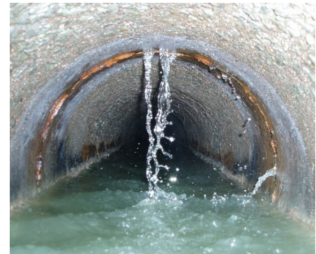
Infiltration into a Sanitary Sewer
