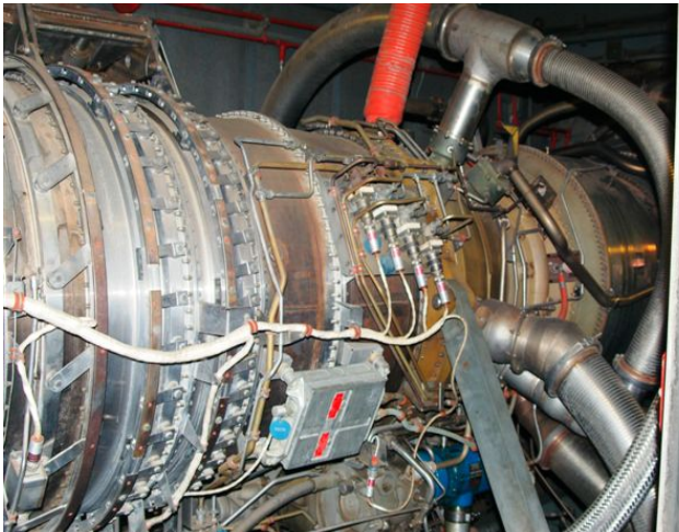
Close-up view of one section of the core of the turbine
